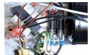
Transformer and fuses.
